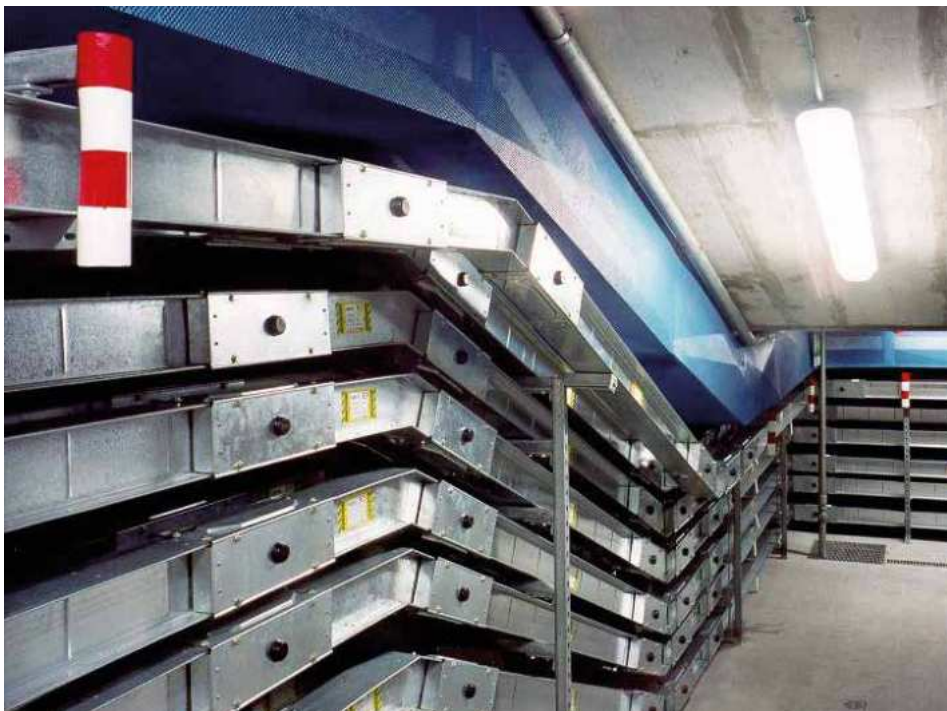
Example of high power distribution
