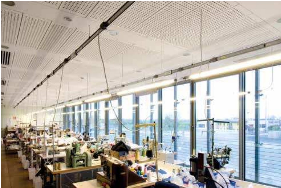
Example of lighting and small power distribution
