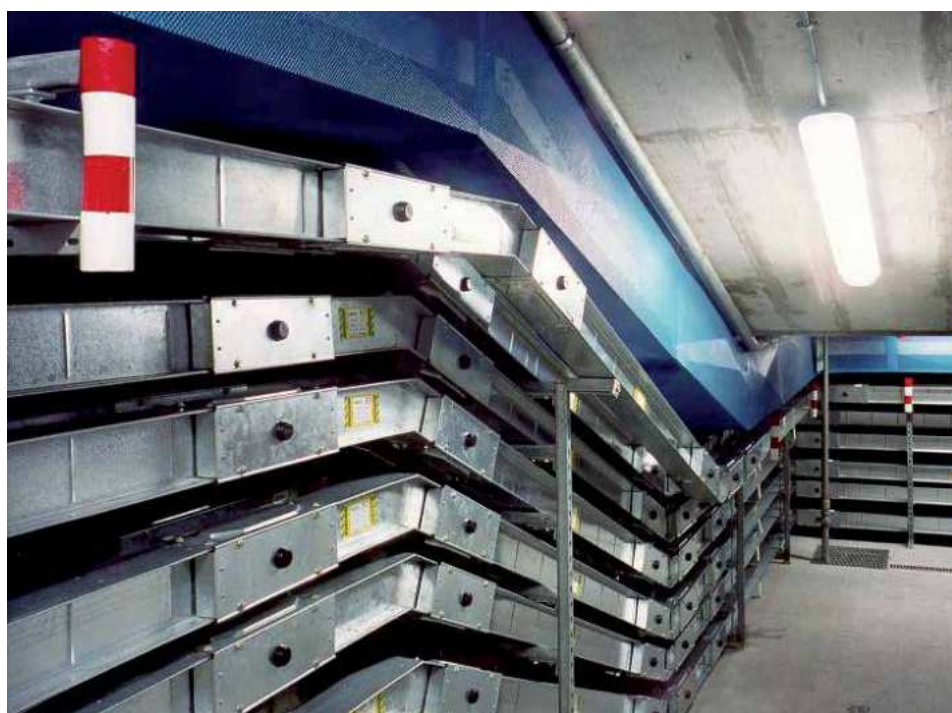
Example of high power distribution
